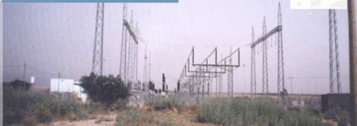
Gaza North substation
